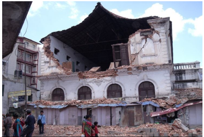
Damaged popular Historic school at the centre of capital
